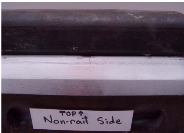
Figure 1. Cracked Joint Bar
