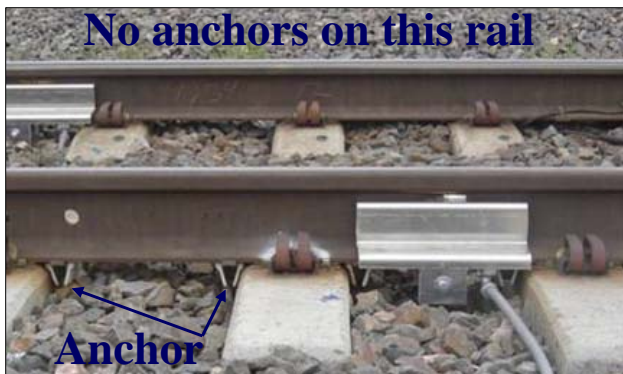
Figure 3. Rails with and without Anchors at Western Mega Site
