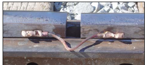
Figure 4. Thermite Welded Track Wire Bond
