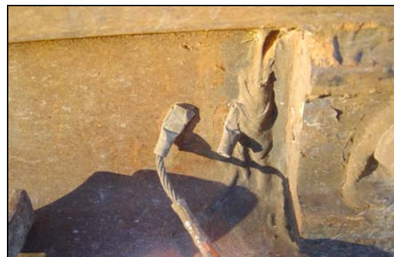
Figure 5. Pin Brazed Track Wire Bond
