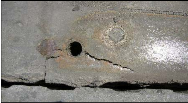
Figure 5. Spike Hole Cracking in Plastic Crosstie
