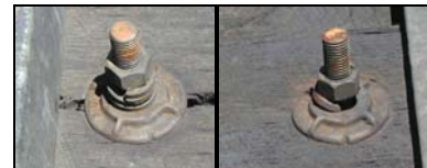
Figure 7a (left). Locking Nut, Spring Lock, and Washer. Figure 7b (right). Broken Spring Lock on Hook Bolt
