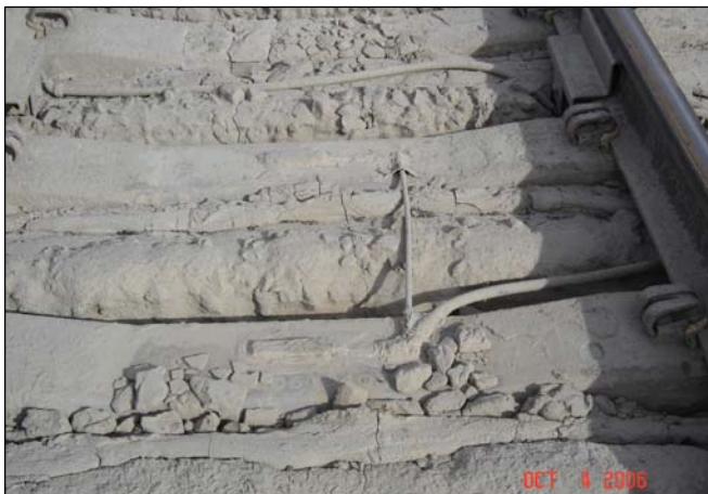
Figure 3. Mud Pumping Holes in the Approach
