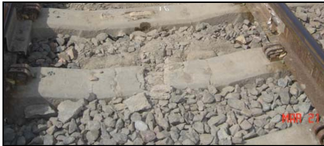
Figure 6. Severely Cracked Concrete Tie
