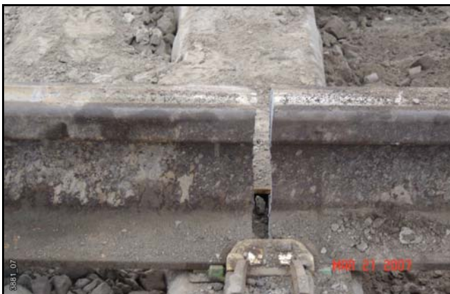
Figure 4. Broken Rail that Occurred in a Mud Pumping Hole
