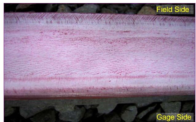
Figure 7b. Post-Grind Rail Surface Conditions, Control Zone (Low Rail — Curve R, Site 1L)
