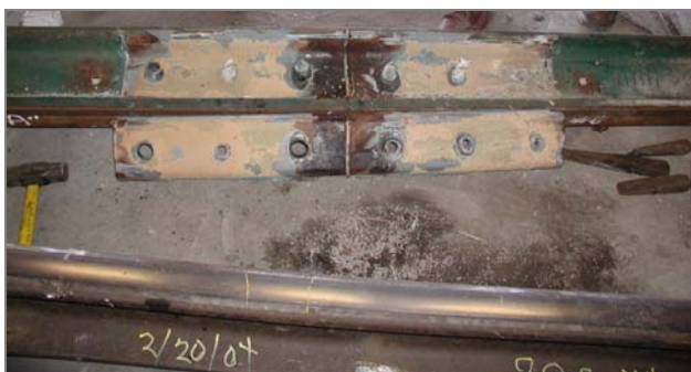
Figure 1. Failed IJ Removed from Service showing Degraded Surfaces
