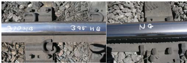
Figure 2. Condition of Unground Rails after 515 MGT. Low Rail Left, High Rail Right
