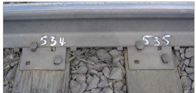
Figure 4. Two Southern Yellow Pine Parallel Strand Lumber Ties Treated with Copper Naphthenate. Tie No. 534 Treated with CPT-2 Solvent. Tie No. 535 Treated with BWR-5 Solvent Appears to have a Thicker Protective Layer and Experiencing Less Tie Plate Cutting
