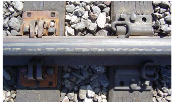
Figure 2. Right Tie: Cut Spiked after Two Screw Spikes Broke Off Inside the Tie. Left Tie: Providing Higher Track Strength with All Four Screw Spikes in New Holes
