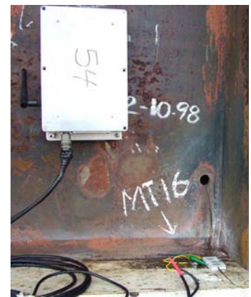
Figure 2. PDL and Sensors Installed at Location MT 16
