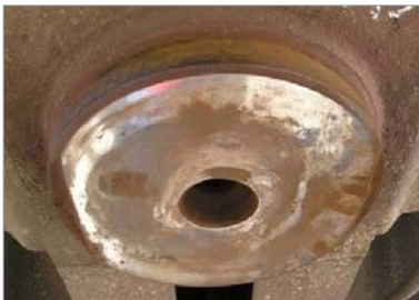
Figure 9. Concave Center Plate Showing Edge Contact and Rust in Center
