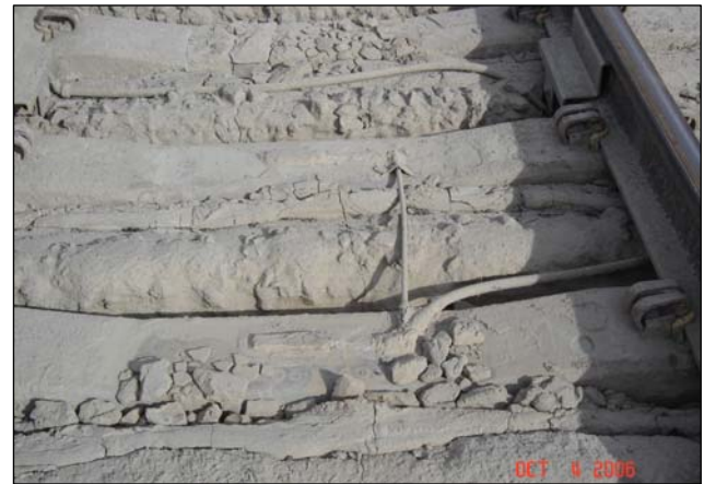
Figure 3. Mud Pumping in the Approach
