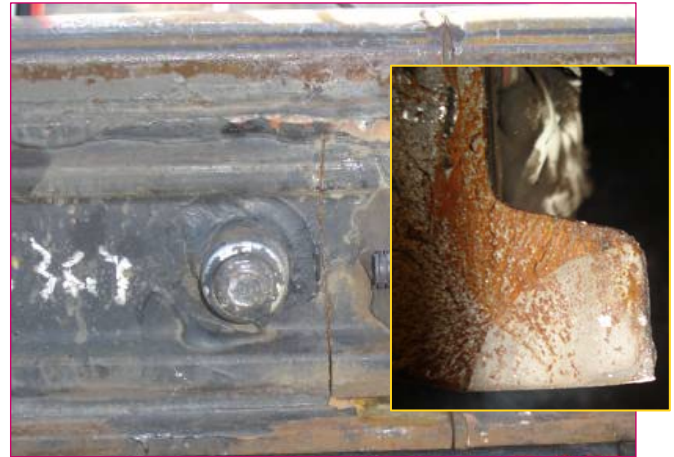
Figure 7. Broken Joint Bar due to Fatigue Crack
