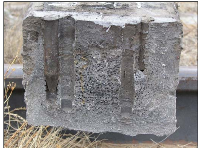
Figure 1. Frog Tie Fractured along the Transverse Plane where Two Sets of Screw Spike Holes Significantly Reduced the Cross Sectional Area of the Tie
