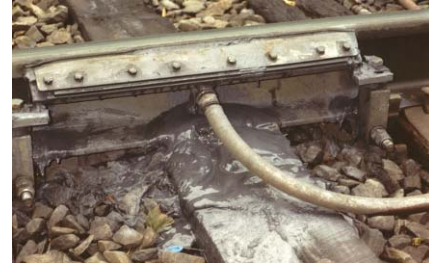
Figure 6. Leaking Bar, FM Material on Tie
