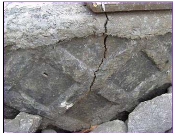
Figure 1. Typical Crack in Rail Seat Area as a Result of Spiking without Pilot Holes
