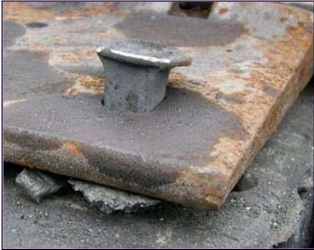
Figure 2. Plastic Material Buildup that Occurred as Spikes were Driven into Ties 1
