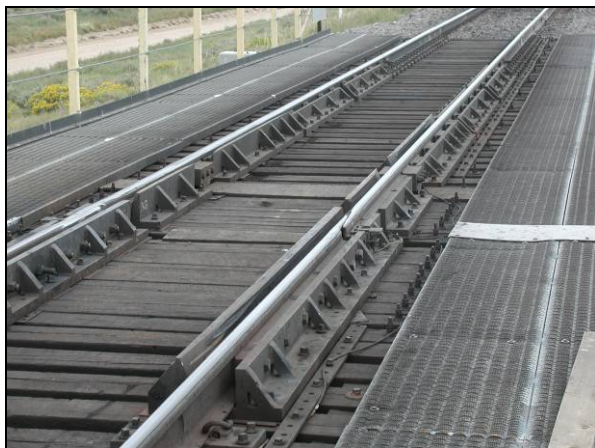
Figure 1: Amtrak Long-Point, Thick-Web Bridge Joints Installed on the Steel Bridge at FAST
