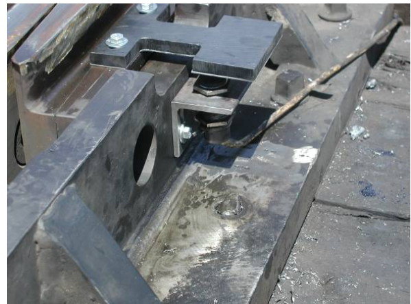
Figure 4: New Delrin Plastic Target and Proximity Switch Bracket Bolted Instead of Welded
