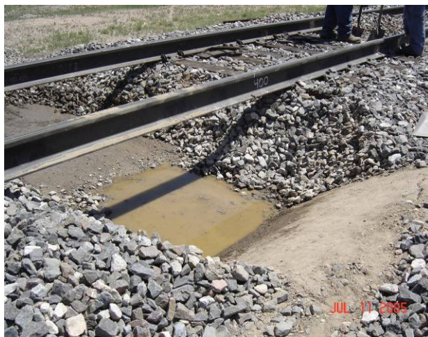
Figure 3. Asphalt Damage and Standing Water
