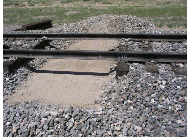
Figure 4. Undamaged Asphalt 210 Feet from the Damaged Asphalt shown in Figure 3
