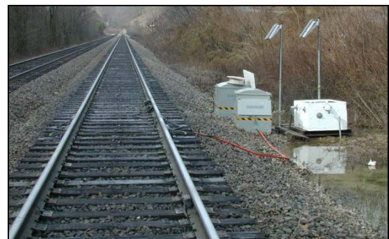
Figure 1. Signal Shunt Monitoring Site and Key Features
