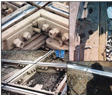
Figure 8. Typical Diamond Crossing Track Degradation
