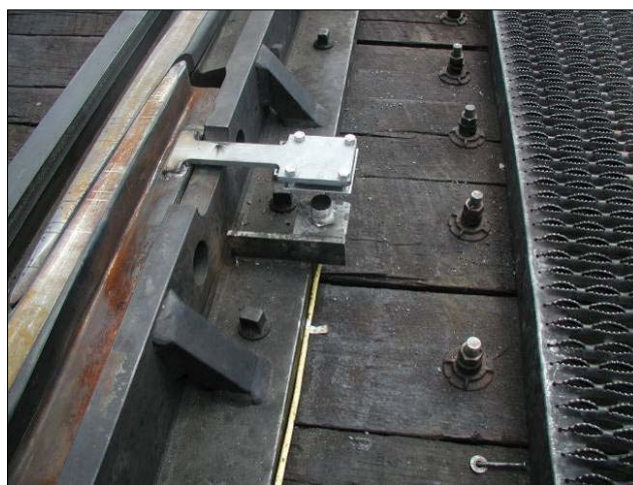
Figure 4: The Second Set of Proximity Switch Brackets
