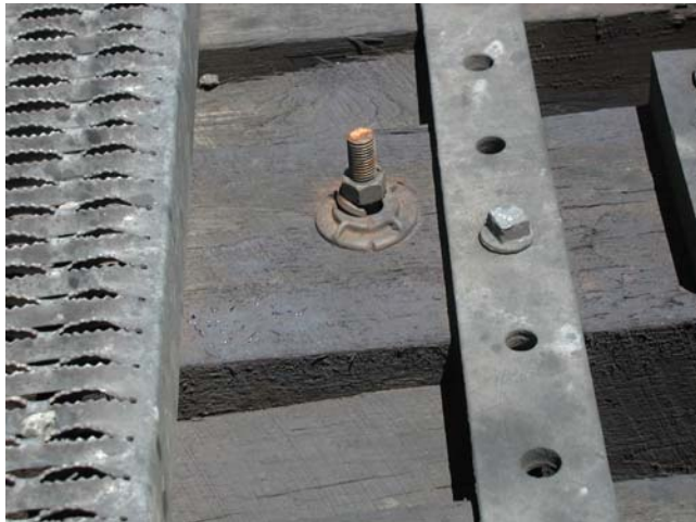
Figure 8: Broken Lock Spring on Hook Bolt
