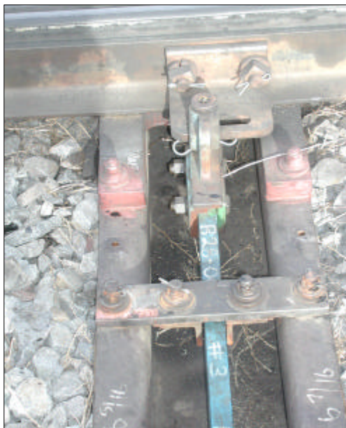
Figure 2: FAST Turnout Switch Rod Binding on Transit Clip and Rod Guides in Cold Weather
