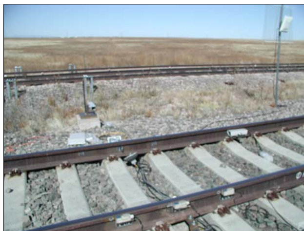
Figure 1. LynxRail ATEX Wheel Profile Measurement System installed at TTC
