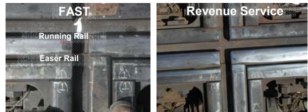
Figure 7. Comparison of Ramped Running Surface Wear Patterns at FAST and in Revenue Service
