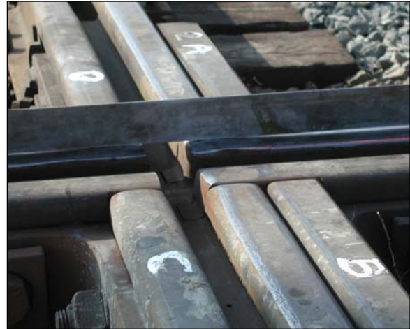
Figure 1. Ramped Running Surfaces after 100 MGT of Traffic
