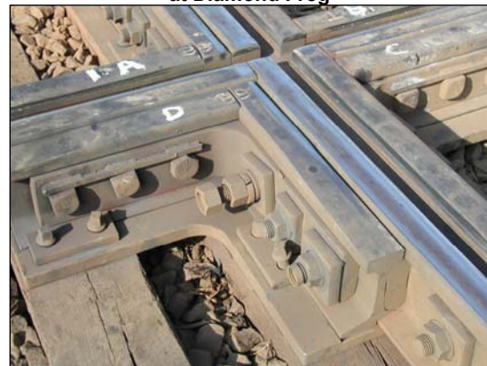
Figure 3. Milled Rail Seat Base Plate (note ¼ inch milled seat at end of easer rail)
