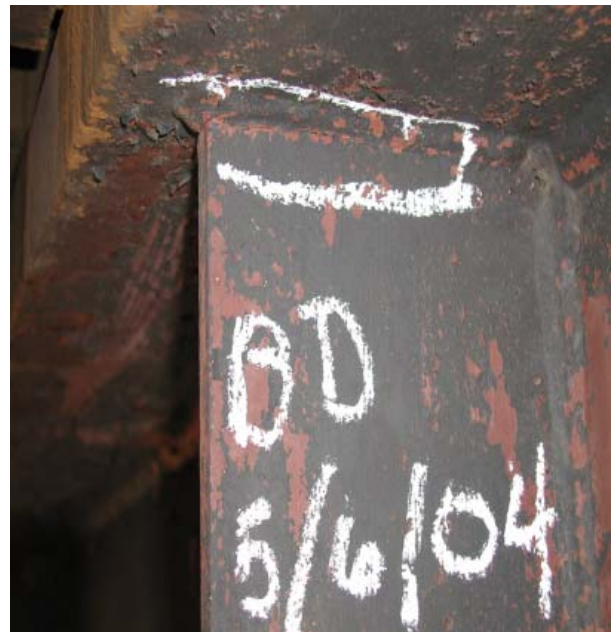
Figure 6. Crack in the Weld of Stiffener and Compression Flange
