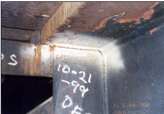
Figure 3. Crack in Diaphragm Connection
