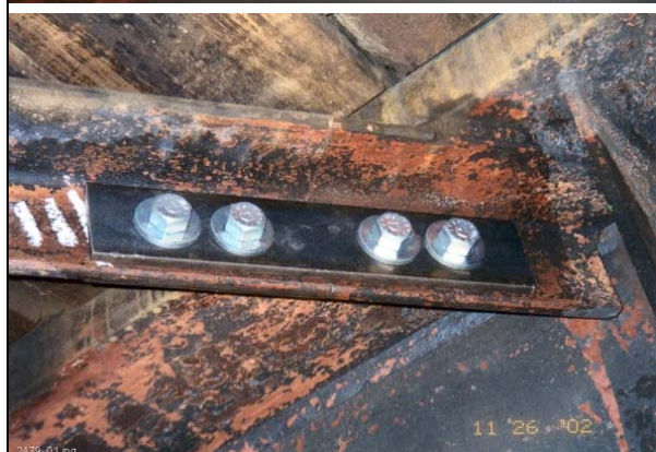
Figure 5. Lateral Bracing (Top) Fractured (Bottom) Repaired with Bolted Splice
