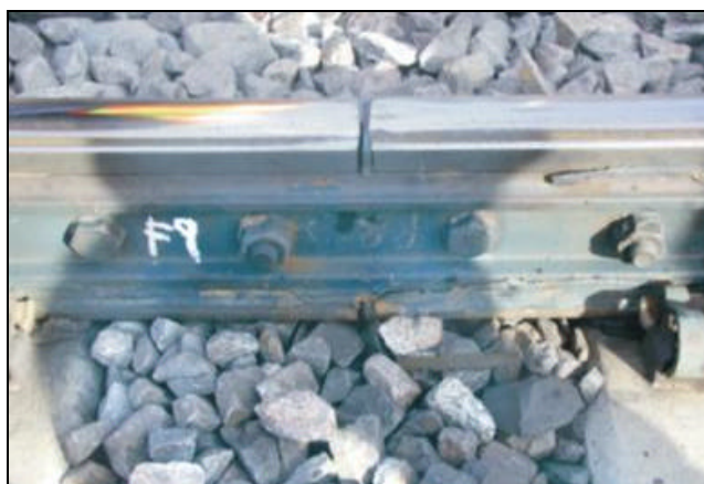
Figure 7. Typical IJ Pull Apart In Track
