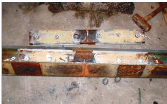
Figure 6. IJ that has Failed-Safe Electrically after Disassembly (Note: Wet areas near end post.)
