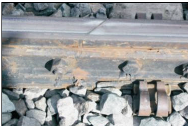
Figure 3. IJ with Running Surface Deformation due to Gap
