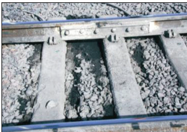
Figure 4. Distressed IJ Foundation in Good Mainline Track
