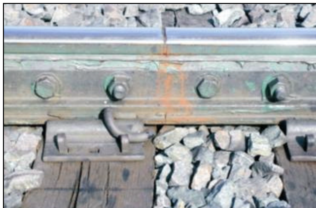
Figure 5. IJ with Glue Bond Fail-Safe Occurrence Near End Post (Note: Rust near end post)
