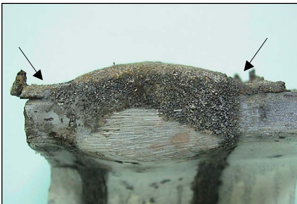
Figure 1: Flashing is present below the rail base on both sides of the weld because the molten thermite portion flowed into spaces that were not completely filled by the mold and/or the sealing sand or paste.
