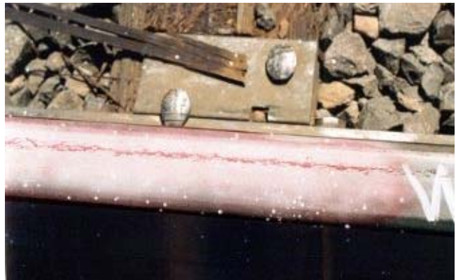
Figure 7. Top of Low Rail, Curve 198A at End of Test after 5 Months near Wayside TOR Applicators
