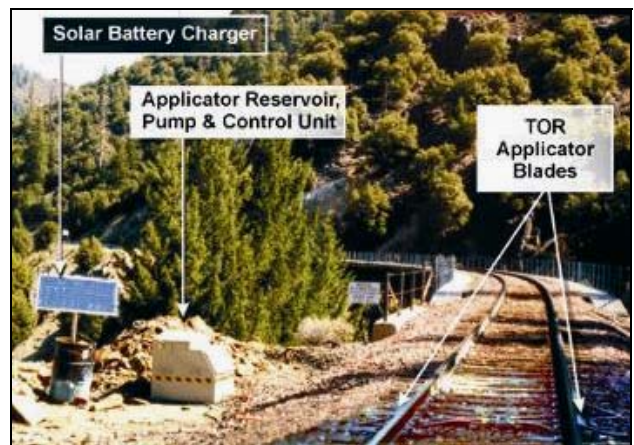
Figure 5. Wayside TOR Application System, Solar Panel and Applicator Bars
