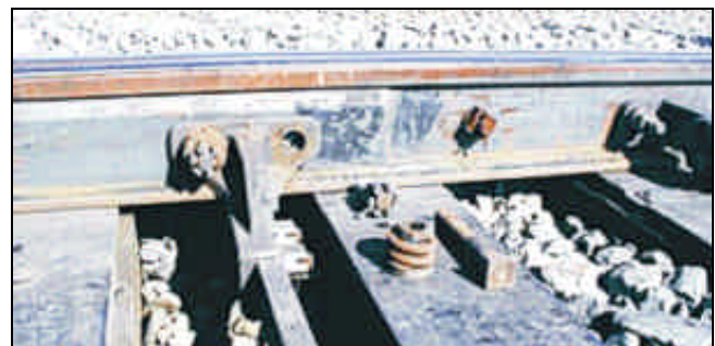
Figure 5. Broken Transit Clip Bolt
