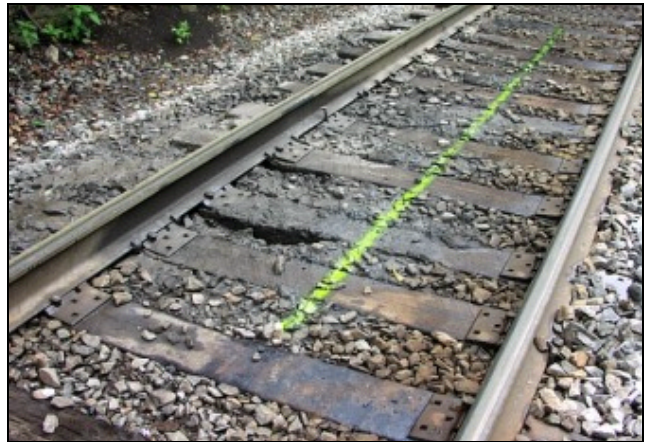
Figure 1. Wide Gage Paint Location at Previous Wash-Out Area in Tangent Track
