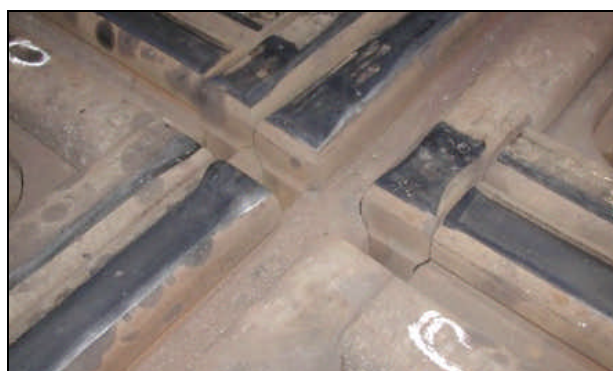
Figure 5. Bainitic Rail Crossing Diamond Common Corner
