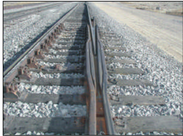
Exhibit 1. Frog No. 3 Installed in Conventional Track
