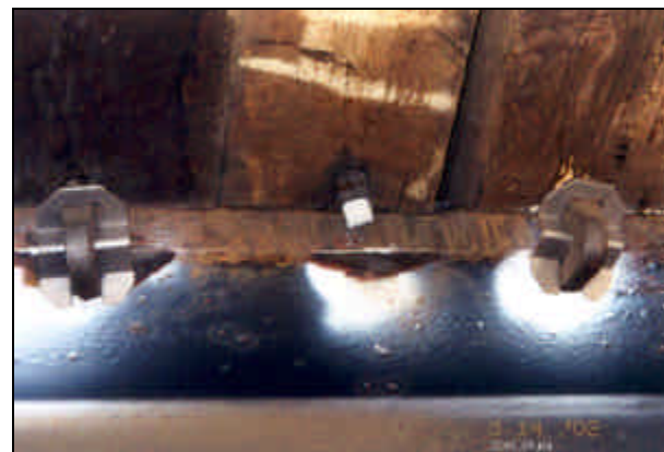
Exhibit 4. Broken Hook Bolt
