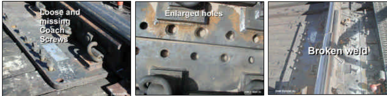
Exhibit 2. Deformed Bolt Holes and Broken Fasteners
