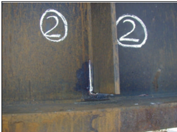
Exhibit 4. Stiffener Weld Toe after Treatment
