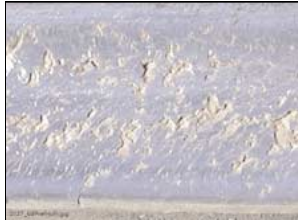
Exhibit 4. Head Hardened Pearlitic Rail from the Inside of the Curve (low rail) Shows Substantial Spalling on the Rail Surface Rail Surface Shown at 110 MGT
