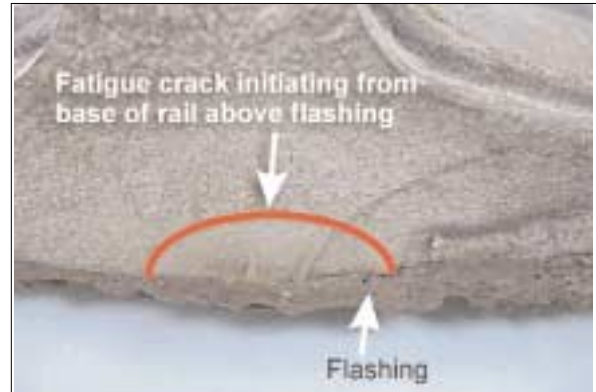
Exhibit 2. Offset Thermite Weld
