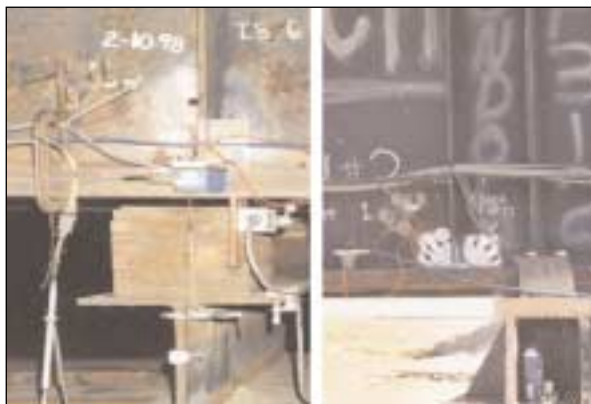
Exhibit 2. Instrumentation at Crack Locations
