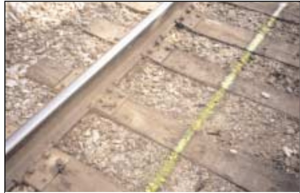
Exhibit 1. Yellow Paint Mark at Site Exhibiting a Broken Spike and Field Side Cant
