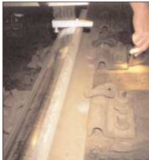
Exhibit 3. Elastic Fastener on an Open Deck Bridge Exhibiting Hidden Plate Cutting
