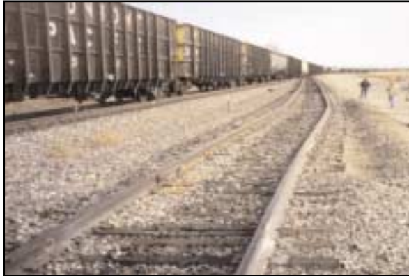
Exhibit 4. Photo of the Buckled Track
