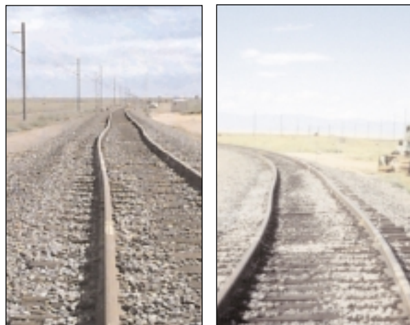
Exhibit 3. Photos Showing Track Buckles
