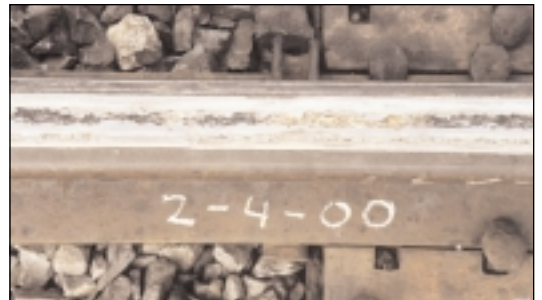
Exhibit 4. Rail Surface Deformation Phases II, III and IV
