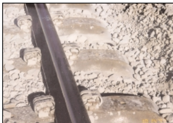
Exhibit 6. Ballast Degradation and Displacement from the High-Side Cribs — Typical Condition Caused by Track Pumping
