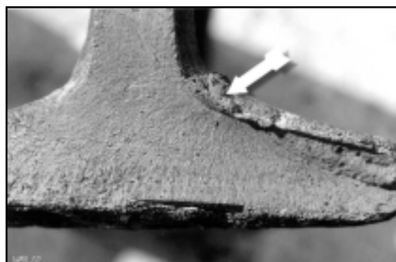
Exhibit 4. Fatigue Defects from Metal Run-Out at Rail Surface
