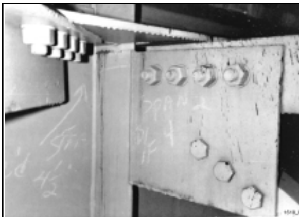
Exhibit 4. Fatigue Crack in Cross Frame, Stiffener and Web Connection
