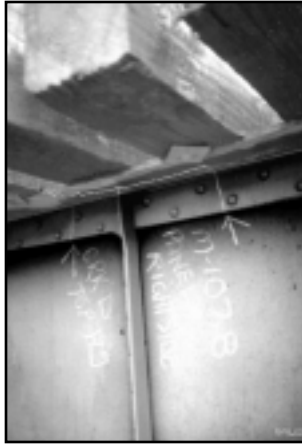
Exhibit 2. Fatigue Crack in the Fillet of Outside Flange Angle
