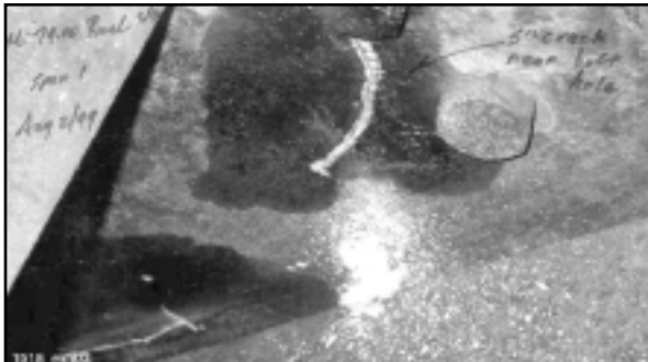
Exhibit 3. Fatigue Crack in Top Flange Initiated at a Bolt Hole
